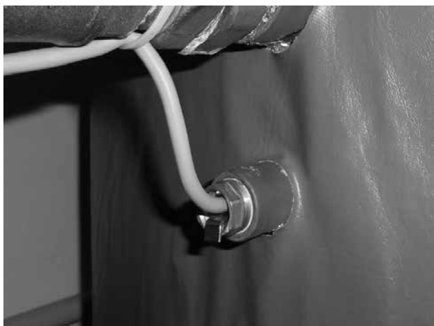
Fig. 13 – View of the water temperature sensor in the pocket of the accumulation tank (TV and TS)
