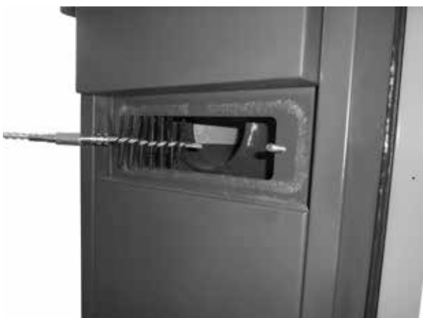
Sample cleaning middle part of the flue way - middle lid
